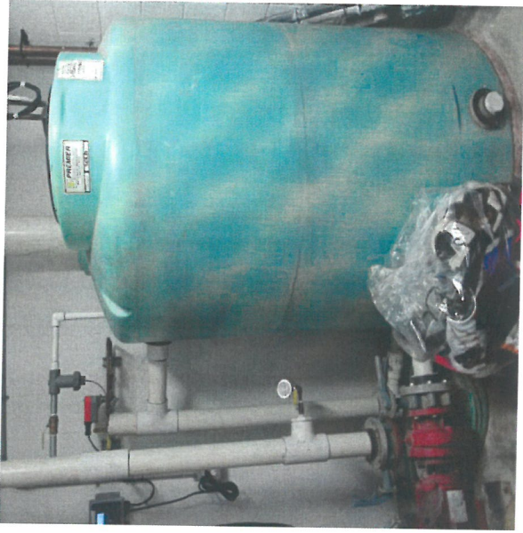
Photo #M10: Brine Tanks.
