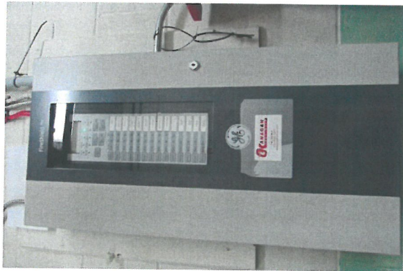
Photo #E9: Fire alarm panel.
