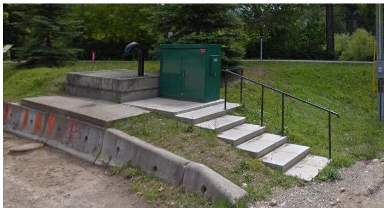
Figure 3-14: Regent Avenue stormwater pumps station
