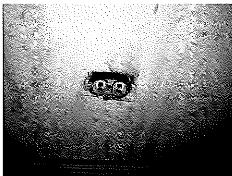
Photo 40: Worn receptacle without cover
