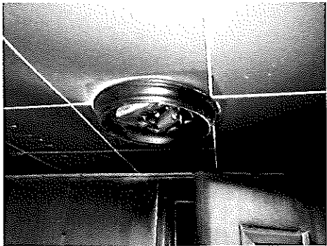
Photo 28: Fixture missing glass and bulbs
