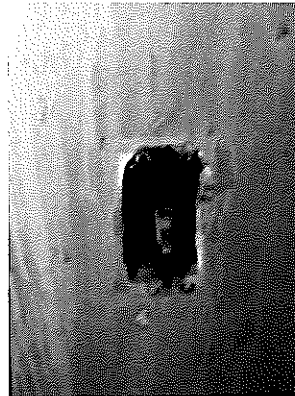
Photo 39: Missing switch cover
