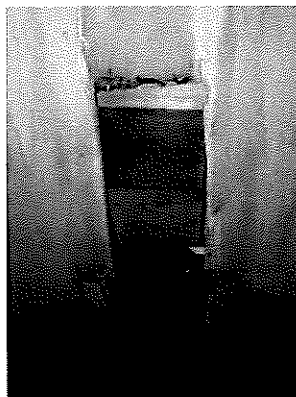
Photo 29: Plumbing access cut in wall
