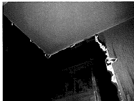
Photo 30: Bedroom 1 closet missing drywall
