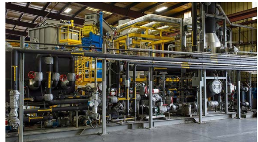
Photo 3: Plastics Pyrolysis Facility
