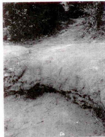
Eby's Hand Launch bank erosion
